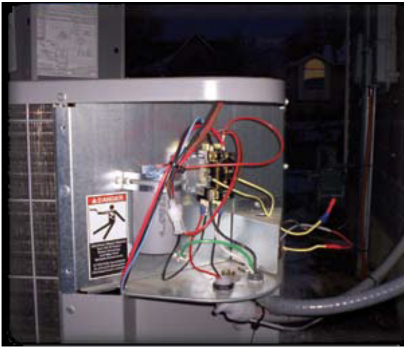
Figure 2: Traditional installation shows DCU wires (bright red, black, and blue) installed at compressor.
